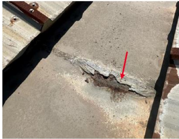
10 Built-in gutter exhibited severe corrosion and section loss at seam locations, typical.
