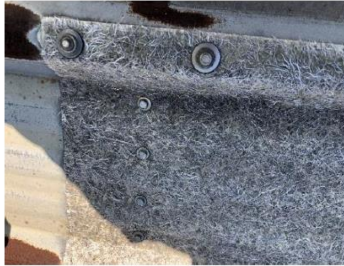
8 Close-up view of fiberglass lite panel; note embrittlement distress.
