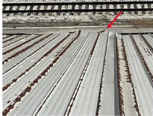
16 Damaged metal roof panel at one location (land side).
