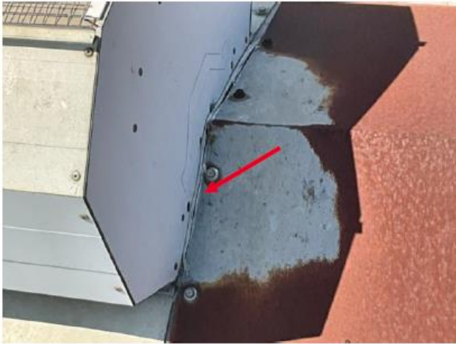
15 Deteriorated joint sealant at roof vent seams.
