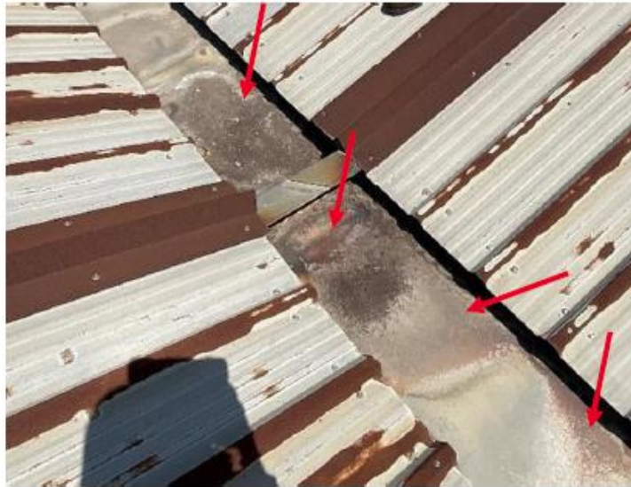
9 Built-in gutter with typical surface corrosion with section loss at seams noted at multiple locations.
