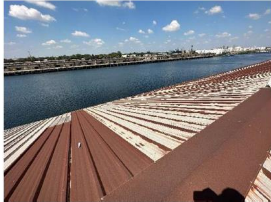
6 Typical View of Metal Roof Panels on the water side with widespread surface corrosion.
