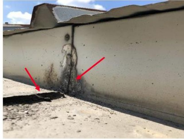
14 Deteriorated joint sealant at built-in gutter seams.
