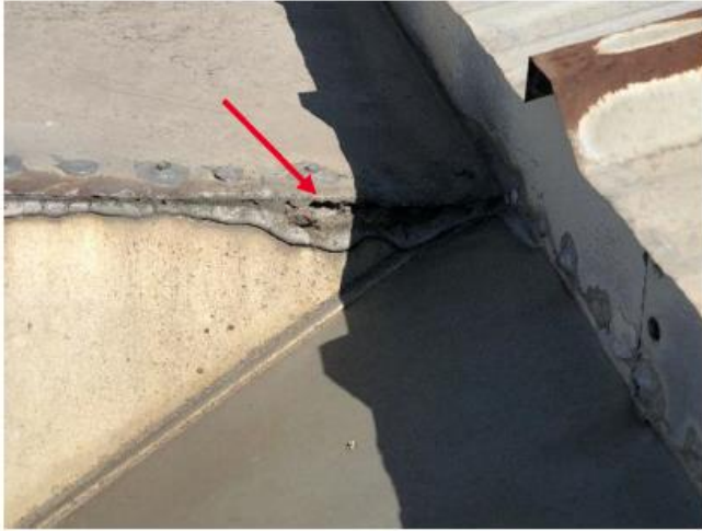
13 Deteriorated joint sealant at built-in gutter downspout inlet.
