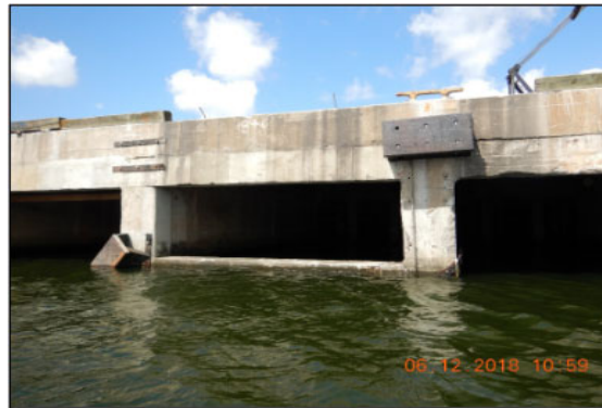
CD48, 1 fender with severe distortion and two missing fenders
