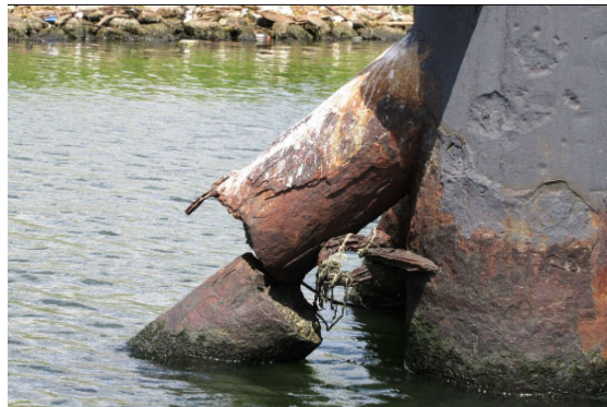
Broken steel batter pile
