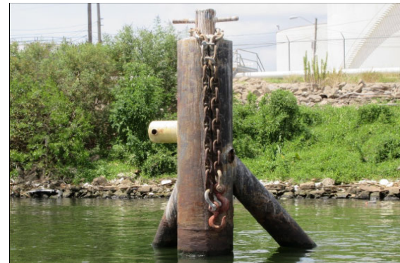
Breasting dolphin missing four fender units
