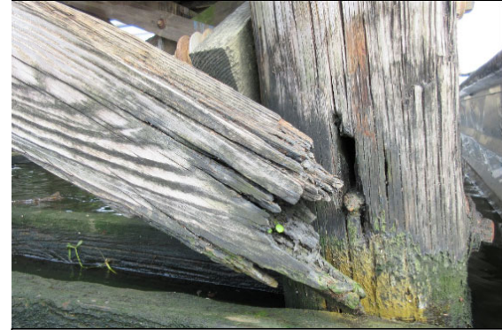
Timber brace with severe decay
