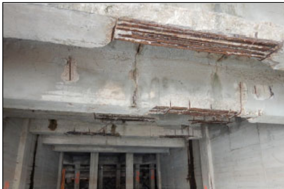
CD48, deck beams with severe cross-sectional loss due to corrosion
