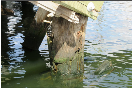
Timber pile broken at waterline
