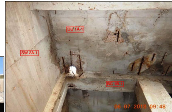
CD47: Bay 1, deck underside with corroded reinforcing and one hole
