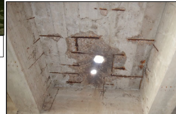
CD48, deck underside with holes and exposed reinforcing with severe corrosion
