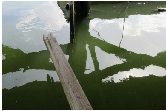
Broken timber brace
