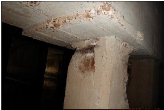
CD47, spalling and deterioration of concrete pile
